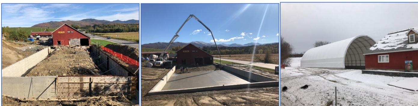
From left to right, site prep work, concrete wall & slab pour and the finished hoop structure.
